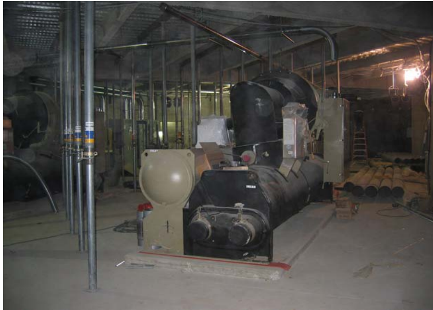
Area 5 Basement equipment room looking west. Equipment set and piping in progress; not yet ready for wiring.
