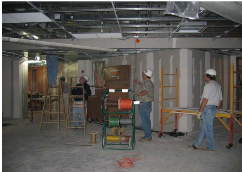
Area 4 Level 2 looking north. Light fixtures installed and above grid wiring in progress.
